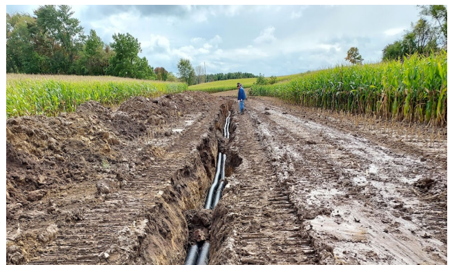
Installation of a water and sediment control basin (WASCoB), a conservation practice designed to reduce erosion, trap sediment, and manage runoff; agricultural field in the Veness Brook sub watershed, Town of Fleming.
