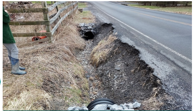
OLWIPD and Tompkins County Soil and Water Conservation District staff identifying severe erosion in a roadside ditch.
