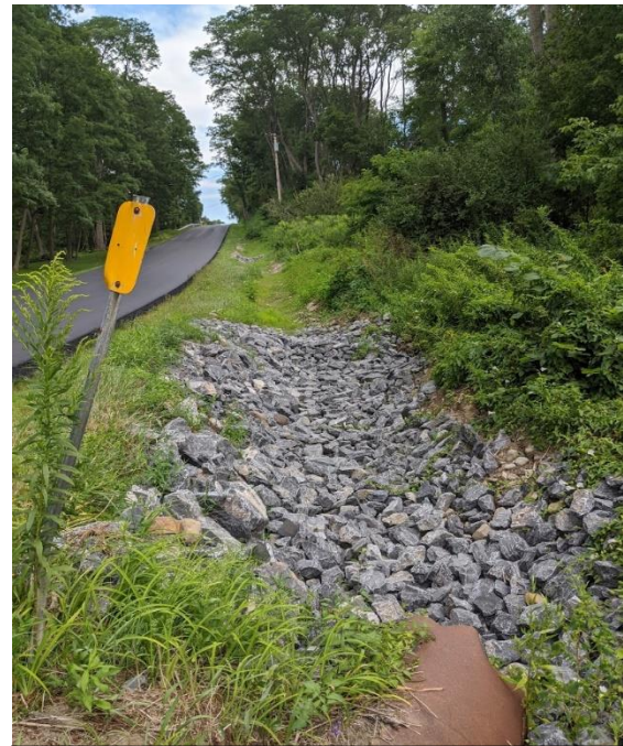
Stone-line ditch, new hydroseeding, and culvert inlet stabilization on West Groton Road, Town of Lansing
